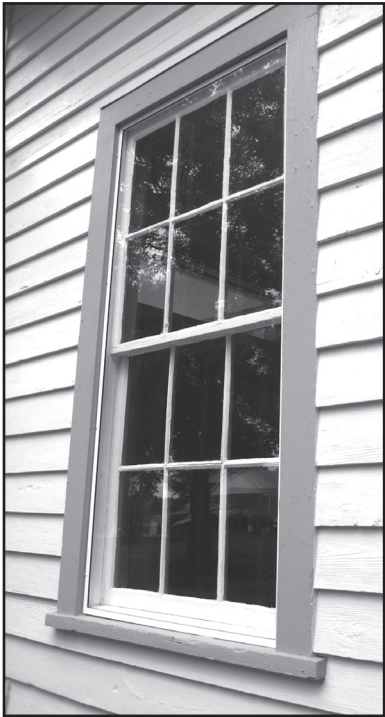
Minimally visible, narrow profile exterior storm windows contribute to the energy efficiency of the Morrisville Christian Church sanctuary.
