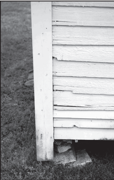
The lower clapboards on this outbuilding have begun to split and crack over time due to weathering and moisture damage.
