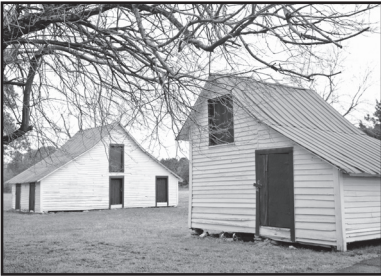
Agricultural outbuildings like these are an important part of Wake County's heritage but are vulnerable to neglect on sites where their function is no longer needed.
